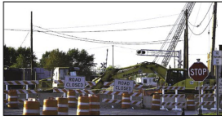
Front Street closed May 4 so that crews can construct an overpass over the two sets of busy railroad tracks.
